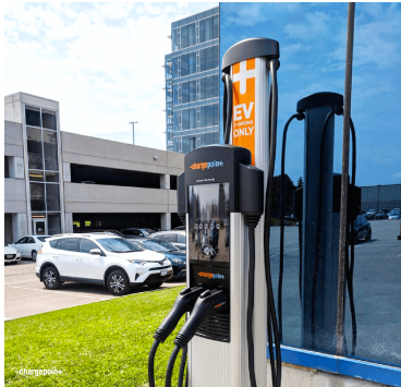
ChargePoint Level 2 EV charger at commercial building
